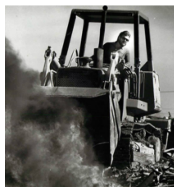
Condominium Destruction (Dallas Morning News Staff Photo by Ken Geiger)
